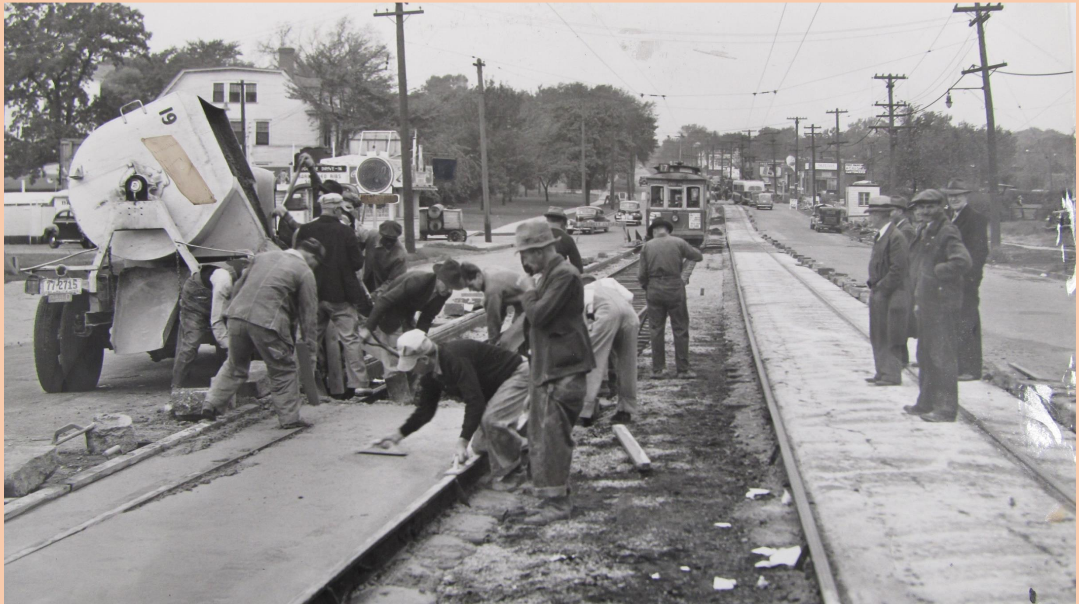
September 1941: WPA workers and streetcar company paving over tracks on Ingersoll east of Harding
